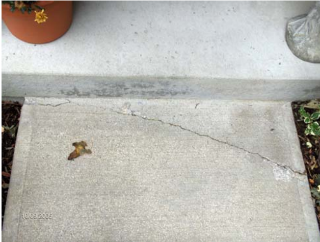
Grounds Figure 6 - Fill/Seal Crack as needed
