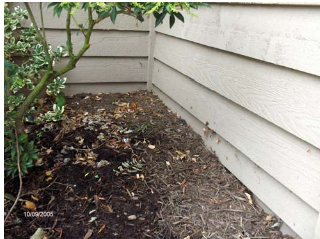
Grounds Figure 6 - Soil in contact w/wood siding
