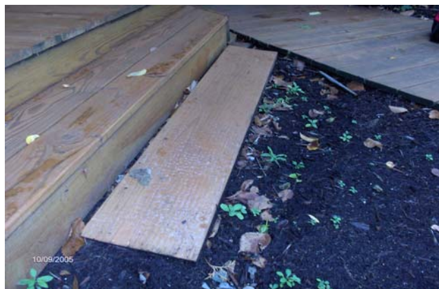
Grounds Figure 6 - Wood in contact w/ soil - watch for deterioration
