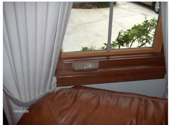
Interior Room 2 - Missing window handels
