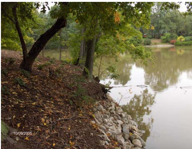
Grounds Figure 6 - Trees close to slope - watch for erosion - remove as needed
