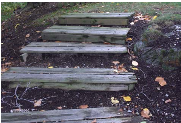
Grounds Figure 6 - Uneven risers - trip hazard
